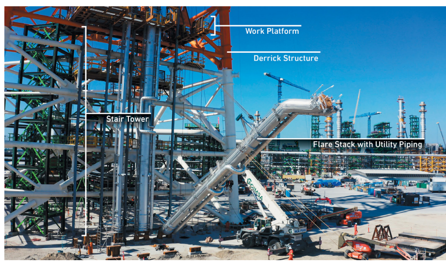
Figure 1. Typical demountable flare system.
