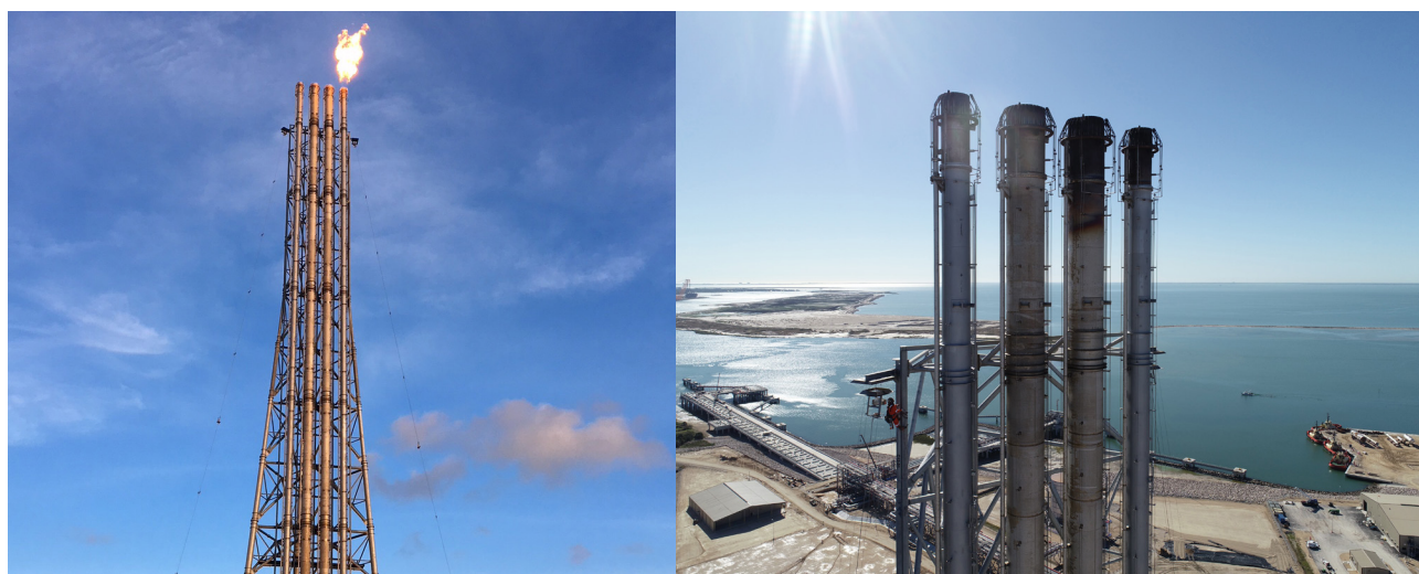
Figure 2. Case study 1 – demountable flare system during operation.
