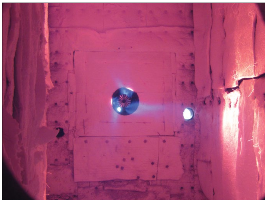
A ZEECO GB low-NO x burner firing 20% CO 2 and 80% H 2 fuel gas.
