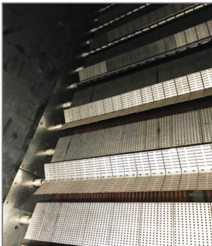
4. This is a look at the completed retrofit of the duct burner system. Courtesy: Zeeco
