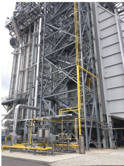
1. A typical combined cycle power plant duct burner system. Courtesy: Zeeco
