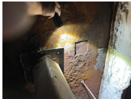
3. This image shows corrosion on the casing wall of the heat recovery steam generator. Courtesy: Zeeco
