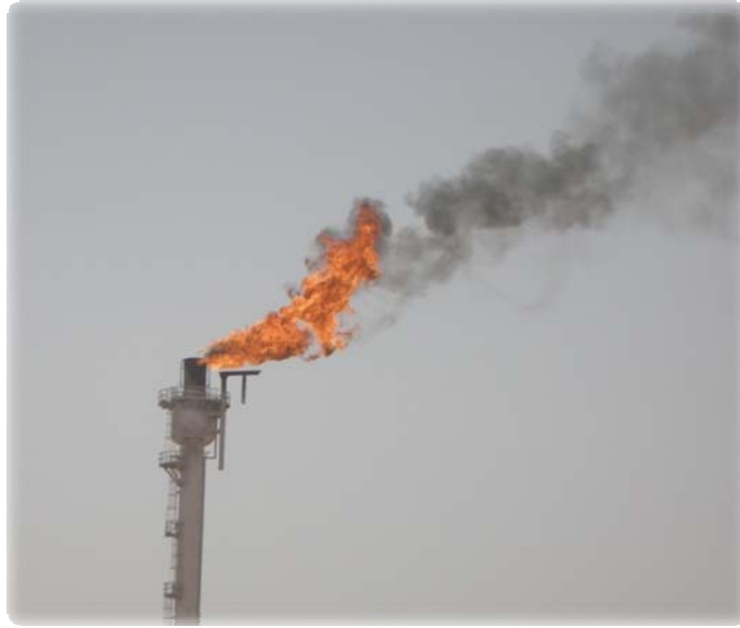
Figure 1. Typical Utility Flare
