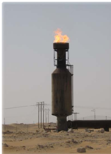
Figure 12. HPAAS Flare Tip at Jobsite D
