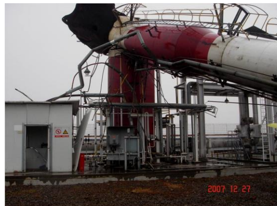
Figure 5. Destroyed Flare Stack as Result of Flashback
