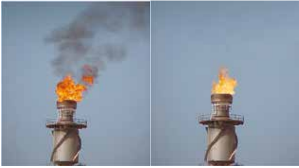
Figure 3. Left: Without HPAAS. Right: The same flare, after retrofitting with HPAAS Smokeless Flare Technology. HPAAS uses supersonic air injection nozzles to inspirate combustion air at a much higher efficiency than any previous air assisted smokeless flaring technology.
