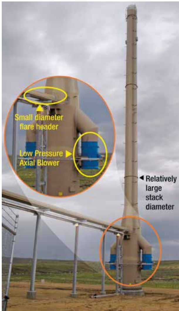
Figure 1. Typical air flare configuration.
