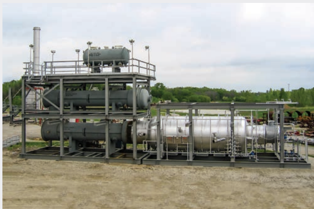
Sulfur Recovery Unit
