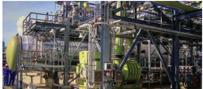
Reaction Furnace Waste Heat Boiler
